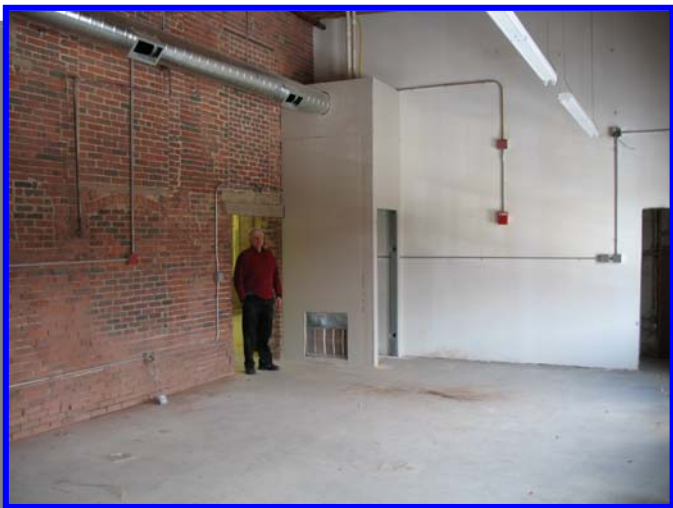
New Heating System
